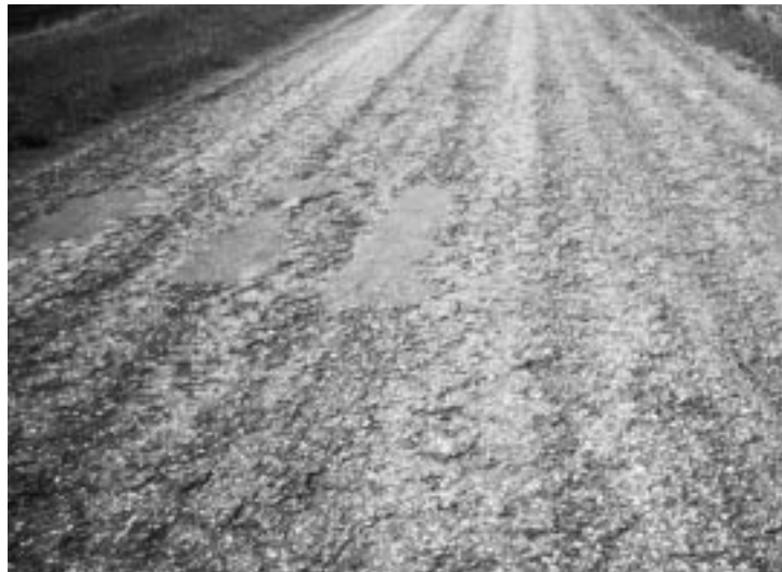
◀ Severe raveling and loss of surface material.
