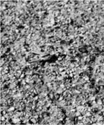
Severe raveling with ▼ extreme loss of aggregate.
