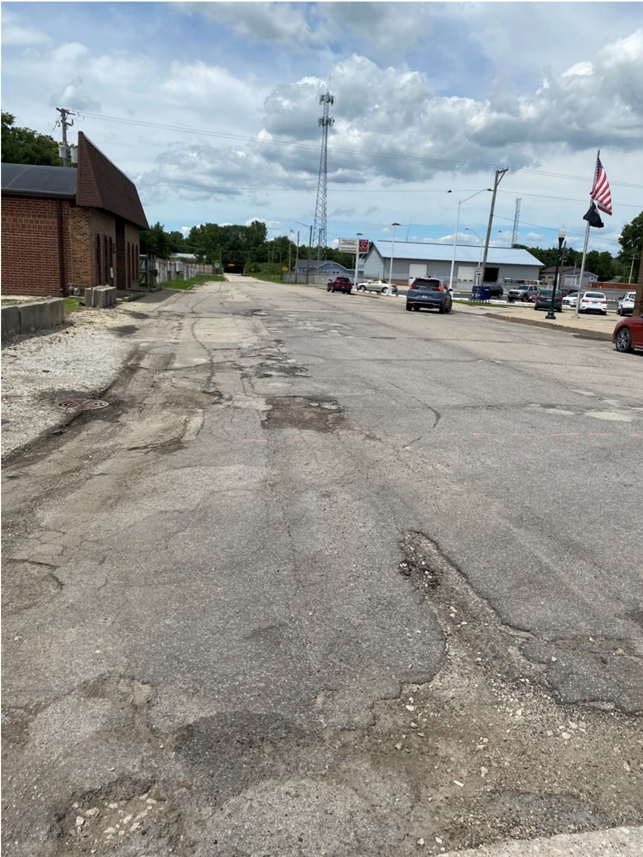
Road Site Pavement Condition 2: Water St. between Van Buren St. and Mill St. (Block Cracking, Potholes, Old Patches)
