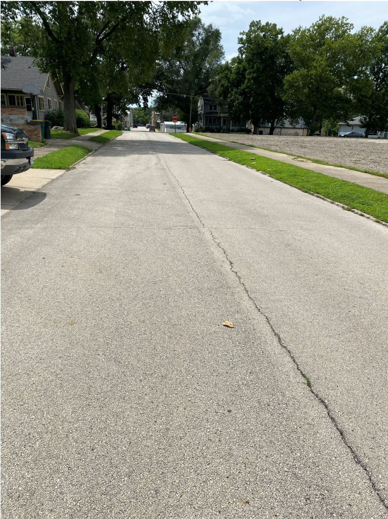
Road Site Pavement Condition 7: Jackson St. between North Kankakee St. and North Joliet St.
