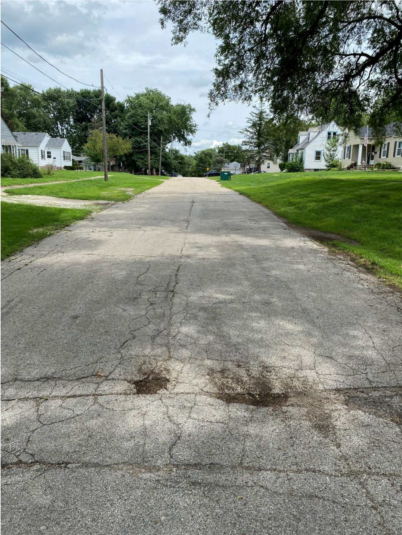
Road Site Pavement Condition 4: Bremer St. between South Washington St. and Milton St. (Block Cracking, Potholes)
