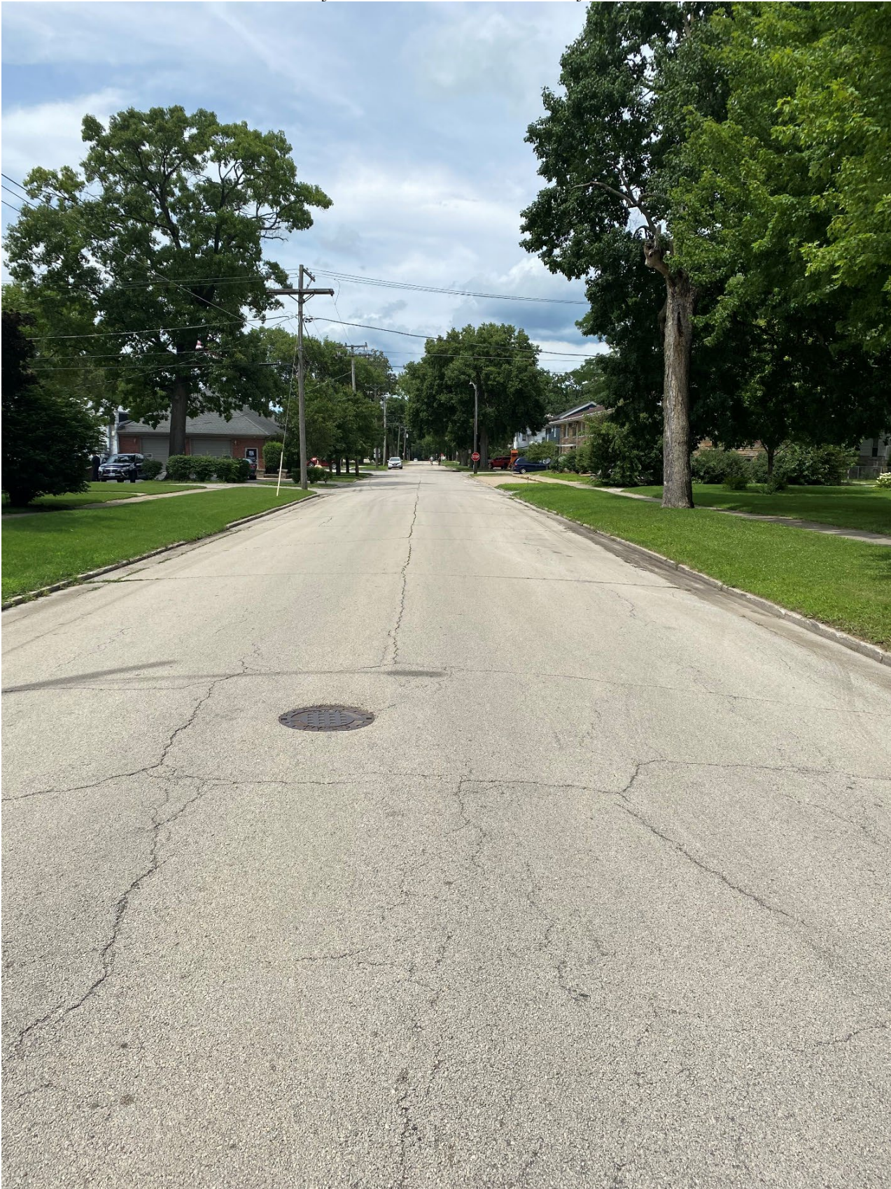
Road Site Pavement Condition 6: South Joliet St. between Route 53 and Jefferson St.
