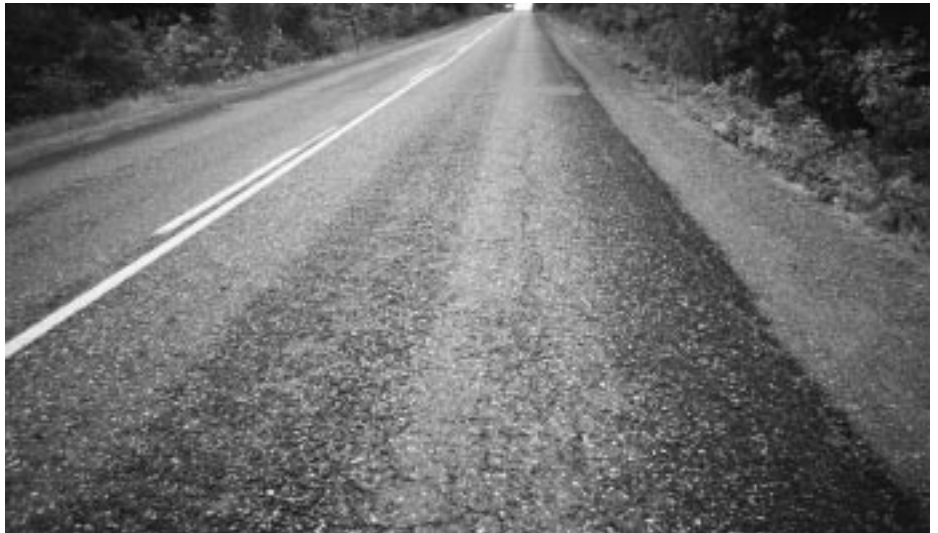
► Moderate to severe raveling in wheel paths.
