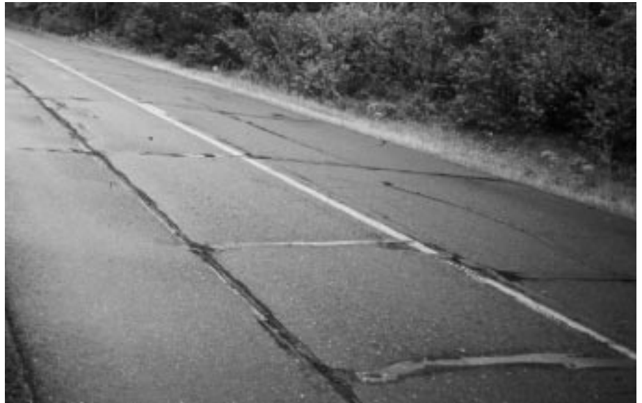
► Concrete joints reflected through bituminous overlay.
