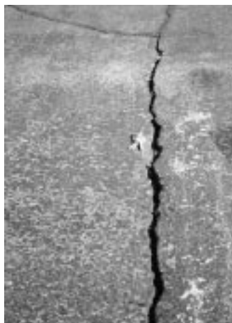
▲ Open crack – 1/2" or more in width.
