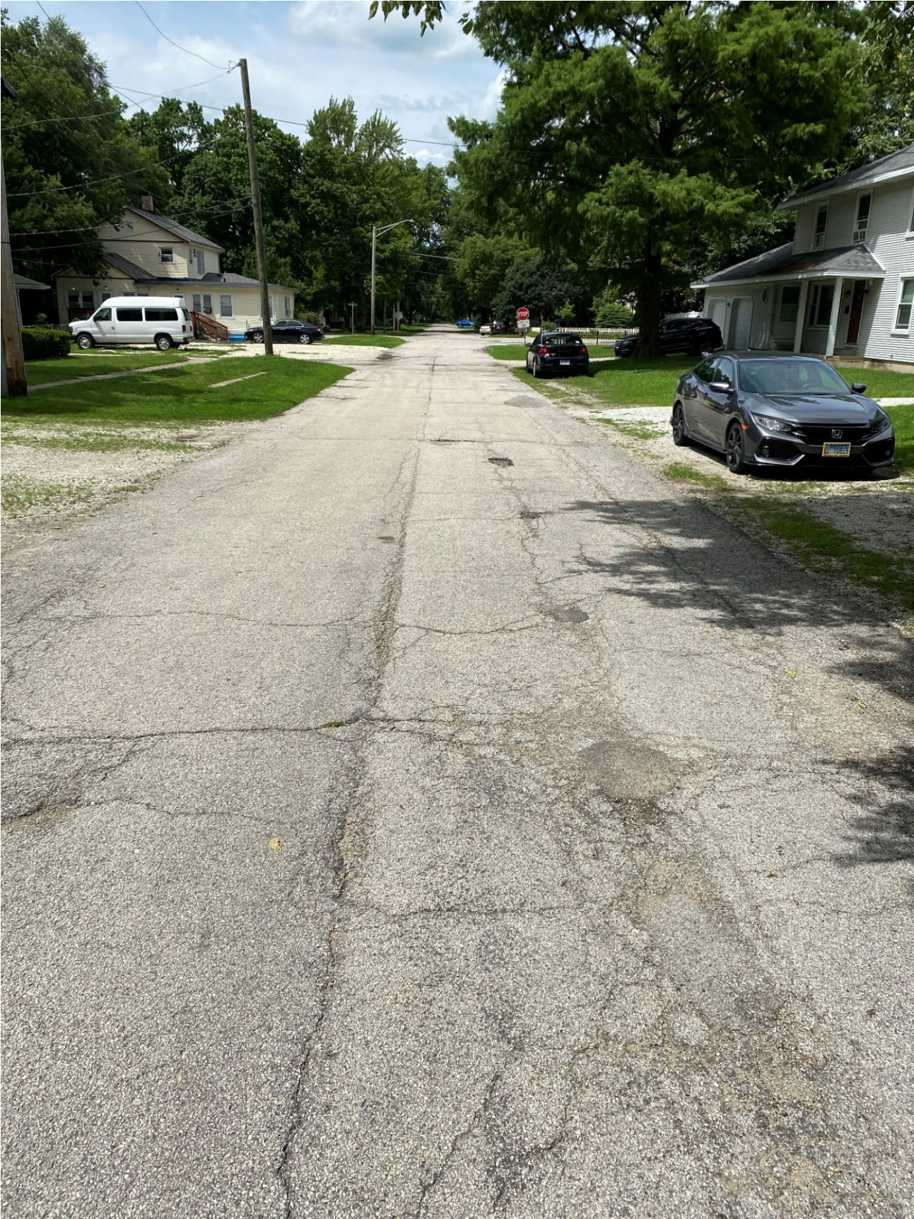
Road Site Pavement Condition 3: South Washington St. between Rte. 53 and Jackson St. (Potholes, Cracking)
