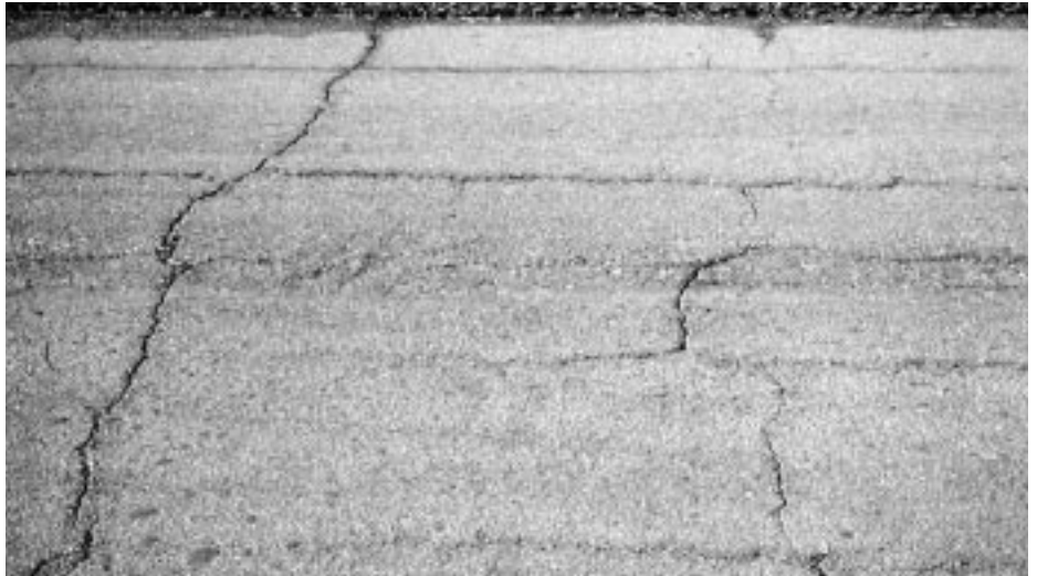
▼ Block cracking with open cracks.
