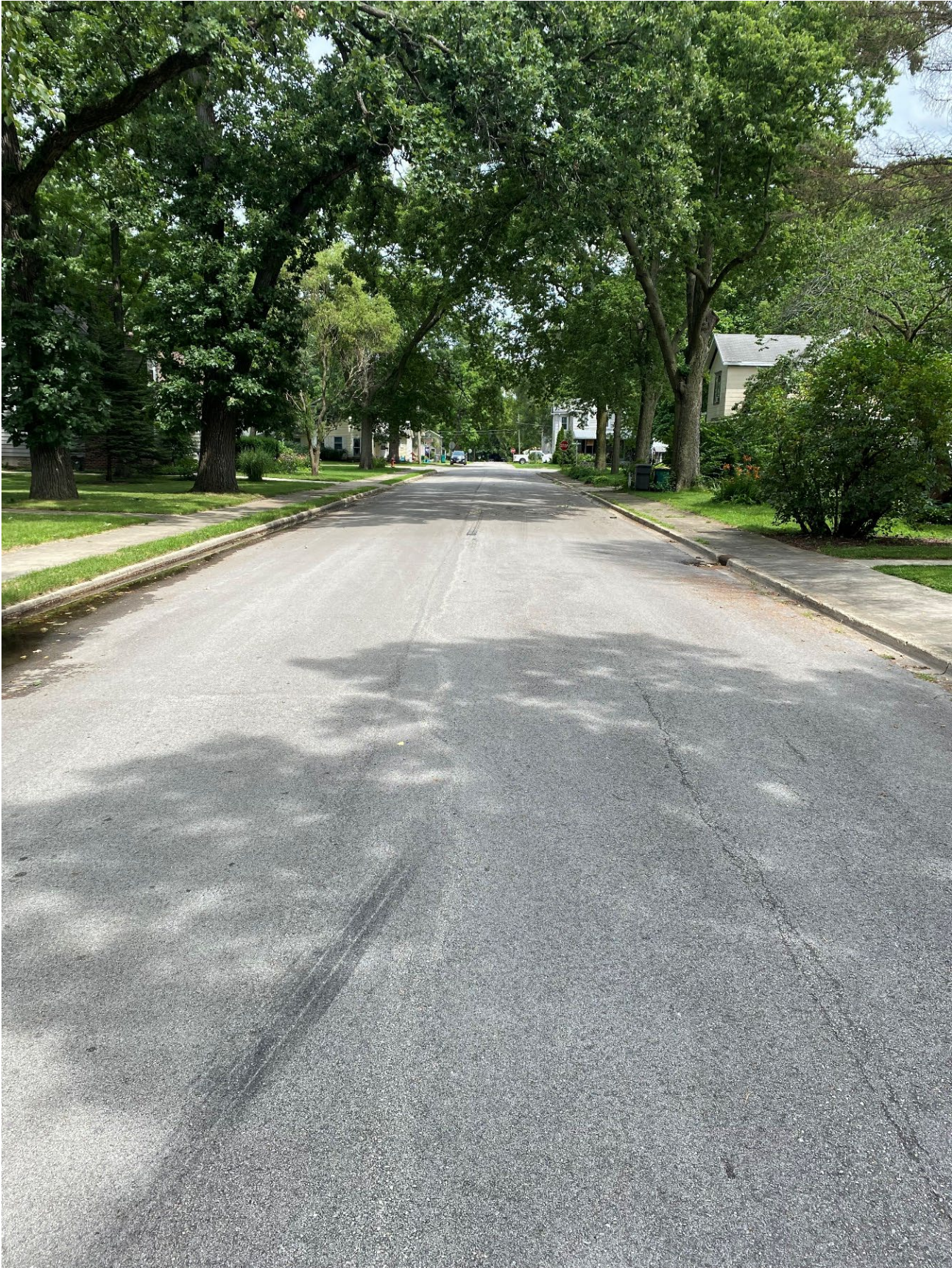
Road Site Pavement Condition 8: Jackson St. between North Joliet St. and Washington St.
