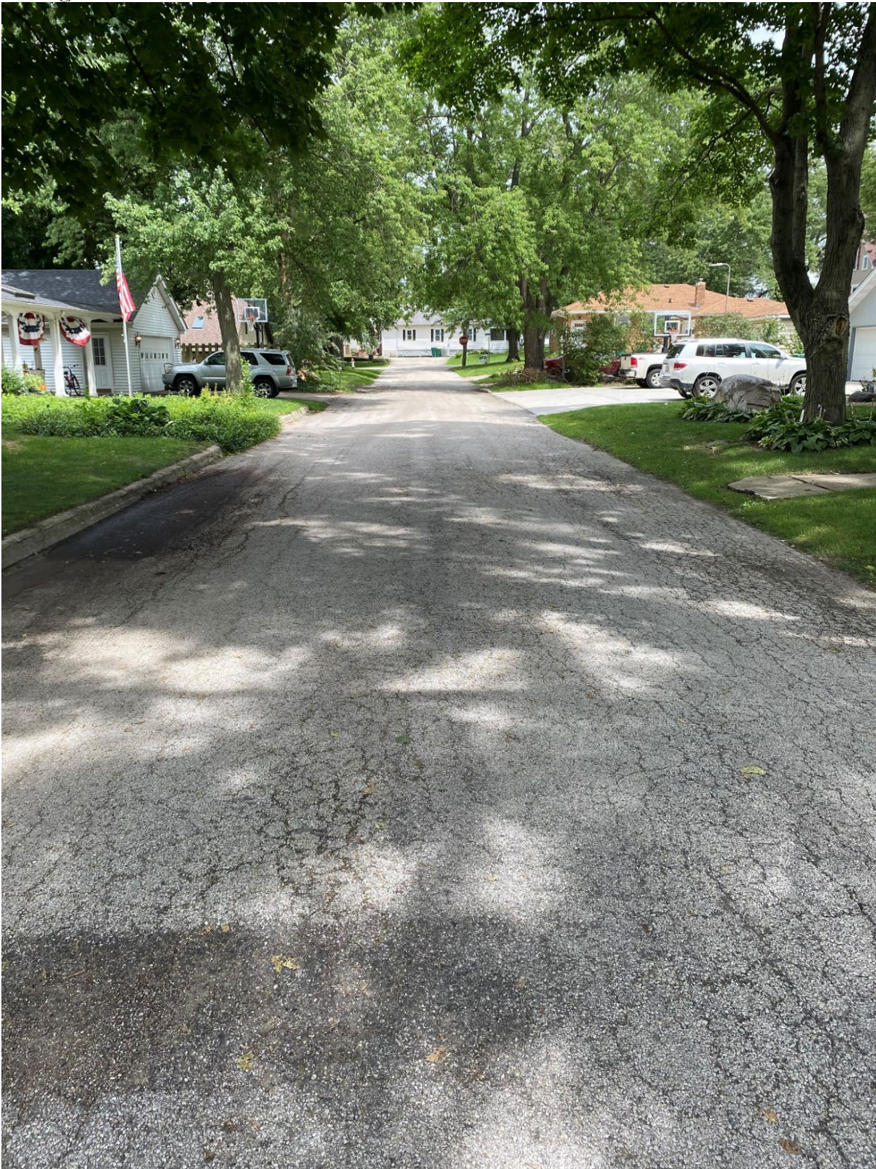
Road Site Pavement Condition 5: Jefferson St. between South Joliet St. and South Washington St. (Alligator Cracking, Raveling)
