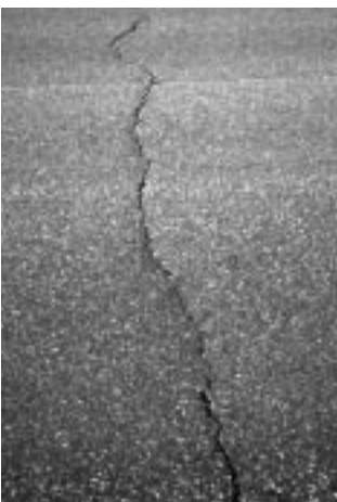
▲ Tight cracks less than 1/4" in width.
