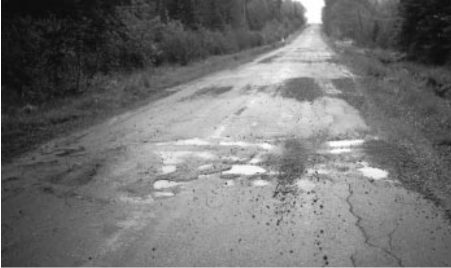
◀ Potholes from frost damage. Reconstruct.
