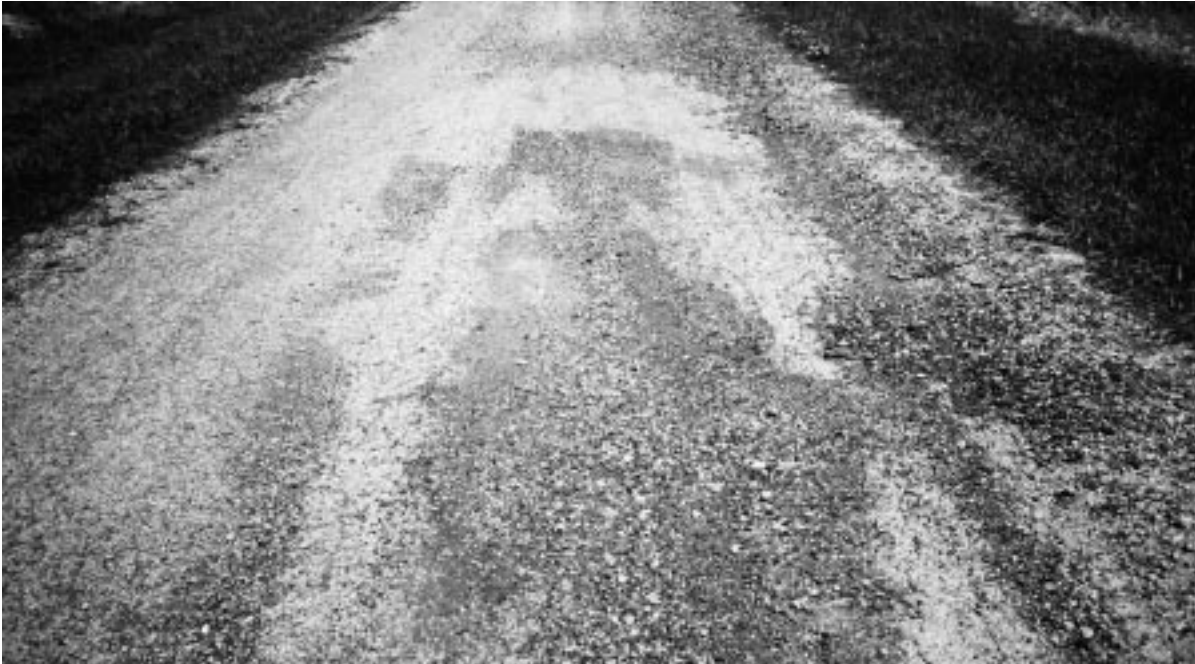
◀ Extensive loss of surface. Rebuild.
